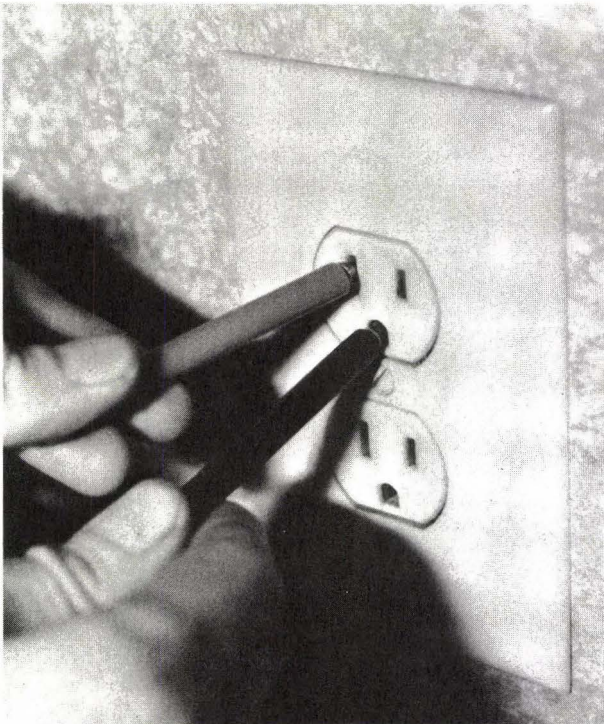
FIG. 6-2 Checking an outlet with a meter.
